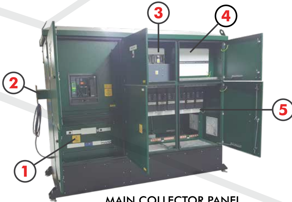
MAIN COLLECTOR PANEL
